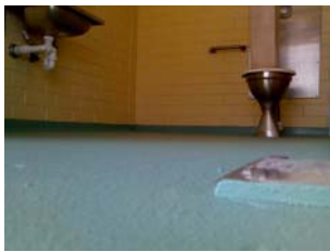
Commercial non slip flooring used to seal & protect the toilet floors at St Kilda playground—St Kilda
