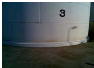
Gripset & Shell combined to seal & waterproof a Sulphuric Acid tank for the ABI group at Pt Adelaide
